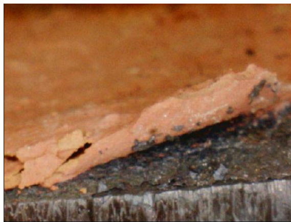
Source: NIST. Figure D-4. Formation of a black scale between paint and steel after exposure greater than 650 °C. Paint readily spalled.
